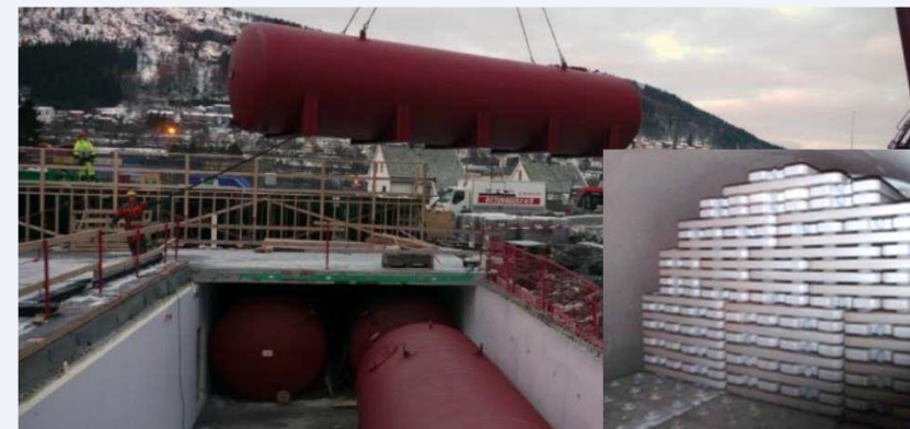
SE; PCM cold storage
